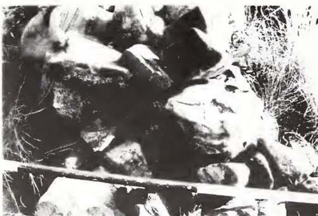
Fig. 9. 2527DC 26 Skeurkloof: construction of the stone wall. Two faces of stone with rubble infill.
